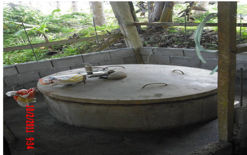
✓ SHALLOW WELL: CAPACITY 3 LPS CENTRIFUGAL PUMP
