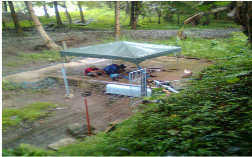
✓ SPRING SOURCE: CAPACITY 15 LPS SUBMERSIBLE/CENTRIFUGAL PUMP
